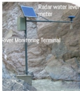
Water Level Monitoring Point (Radar)
